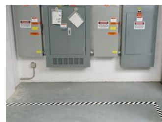
6. Colour-code areas in front of electrical panels.
